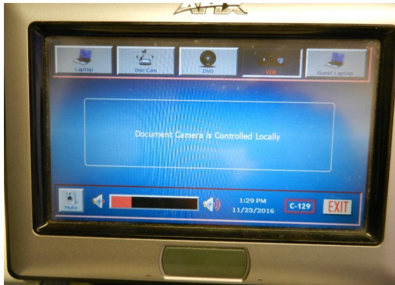
Figure 5: Master Control Panel Main Menu
