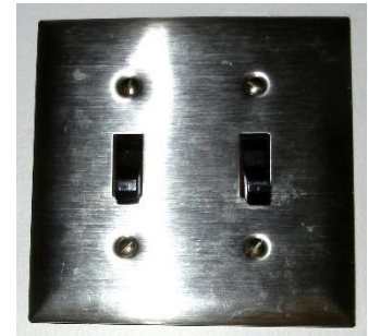
Figure 31: Overhead Lights Switch (Front & Back)
